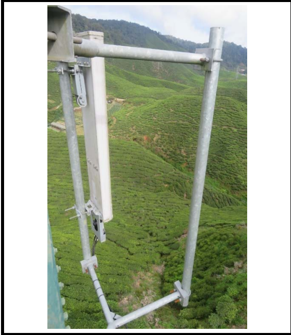
Existing DB HH Antenna (U21) @ 18m AGL, Sector 3
