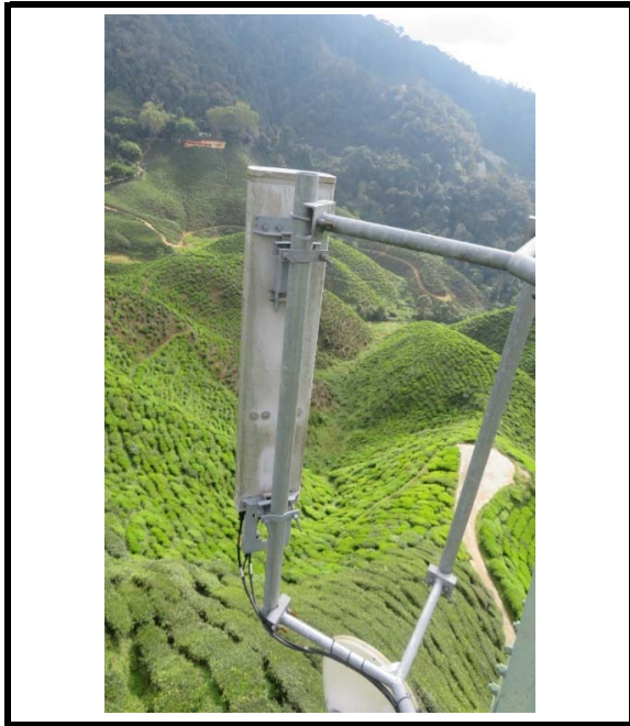
Existing DB HH Antenna (U21) @ 18m AGL, Sector 1
