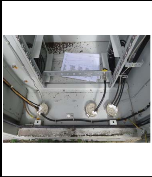
Cable Inlet Location (Inside Room)
