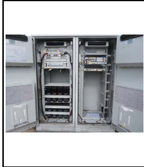
Existing RBS #1 Location (Door Open)
