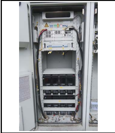
Existing Rectifier Full View #1
