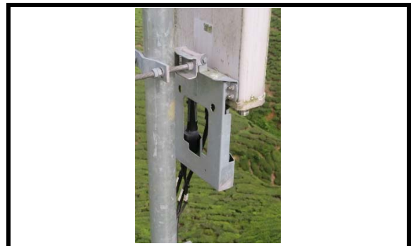
Existing Antenna 1 Port Sector 3
