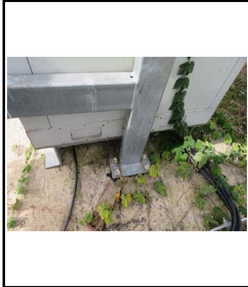
Cable Inlet Location (Outside Room)
