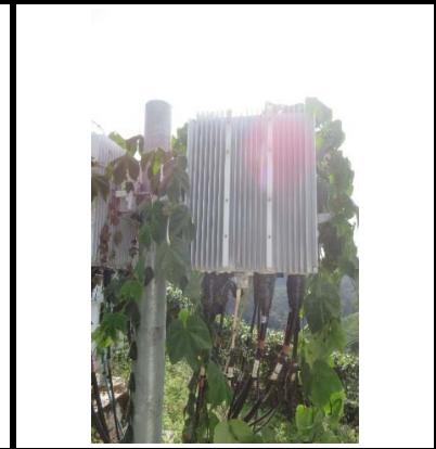
EXISTING RRU S3 U2100
