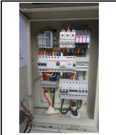
Main ACPDB Breaker
