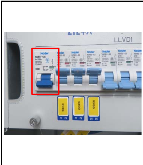
Reused DC Breaker Location
