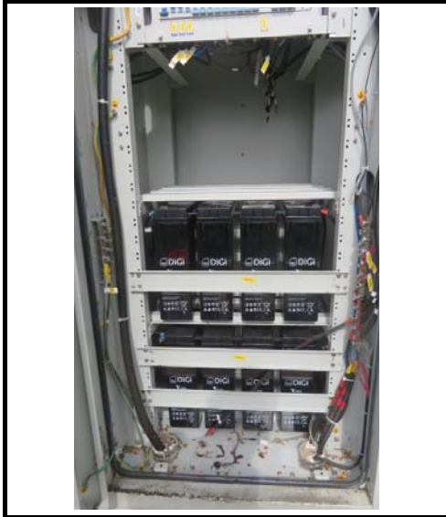
Existing Battery Location
