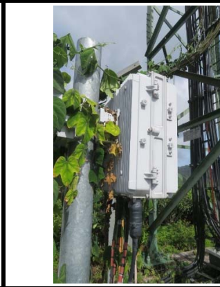
EXISTING RRU S2 U2100
