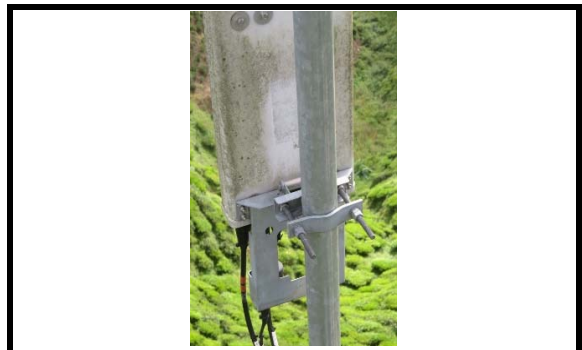
Existing Antenna 1 Port Sector 1
