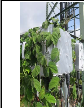
EXISTING RRU S1 U2100
