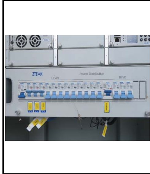
Existing Rectifier Full View (Door Open) #1
